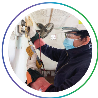
Project "Improving Electrical Safety in Vietnam"
